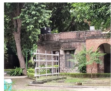
Hydroponics system for grey water recycling
