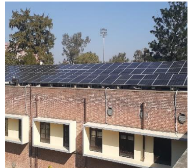
Solar PV installed
