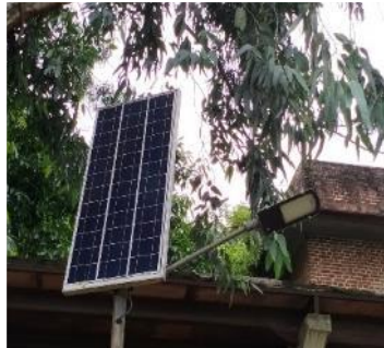
Solar Lights Installed
