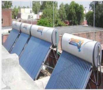
Solar Geyser Installed
