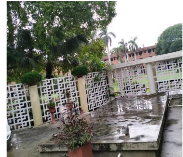
Rainwater Storage Tank
